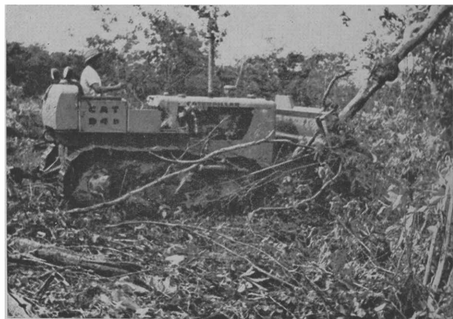
Figure 2. Wet season clearing of a dense brush stand with a bulldozer equipped with a brush hook. The brush was pushed into piles, or windrows, and later burned.
